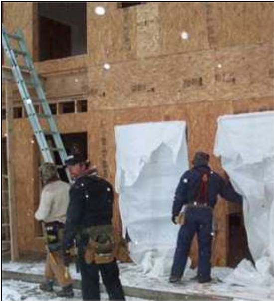
Property owner and builder Paul Montoya checks behind the makeshift snow guard on one ranch project that didn't quite get completed before the first snow.
